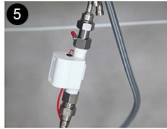
5 The picture above shows the installed touch sensor
