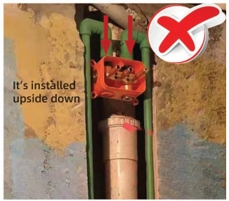
It's installed upside down The installation of concealed plastic box in wrong way
